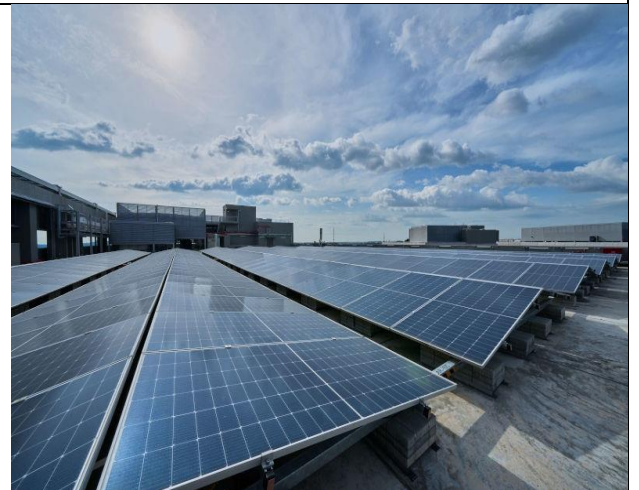
Rooftop solar panel in Punggol
