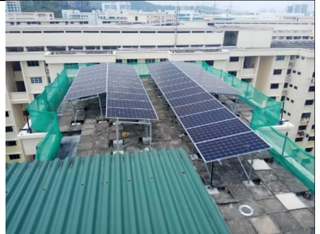
Rooftop solar panel in Bukit Panjang
